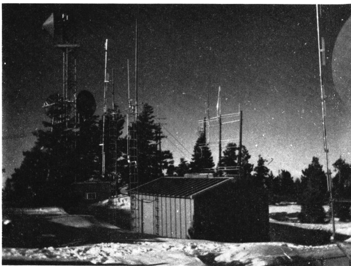
Fig. 1-6. WB6SLR's remote installation at a commercial facility atop 8500-foot Blueridge Summit in California. Equipment is shown in Fig. 1-7.
